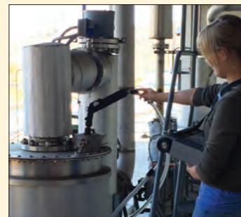
Plant Operator Courtney Hernandez uses the TVA 1000B VOC analyzer to measure the VOC levels of the ozone destruct unit headspace.
