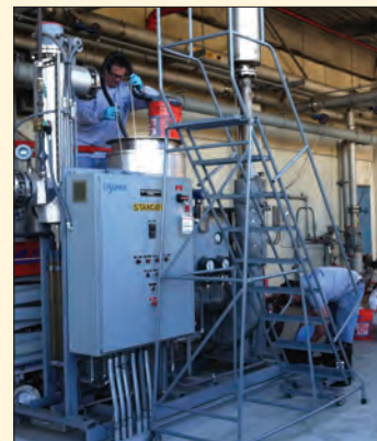
Treatment Plant maintenance staff inspects the ozone destruct unit vessel after removing the catalyst.
